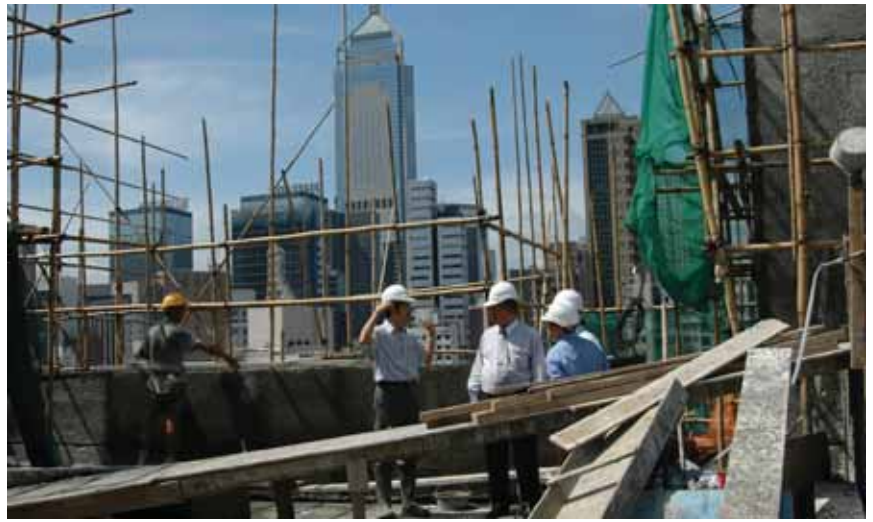
School Principle Mr. George Tam inspected the near completion SIP annex on 1st September 2004.
